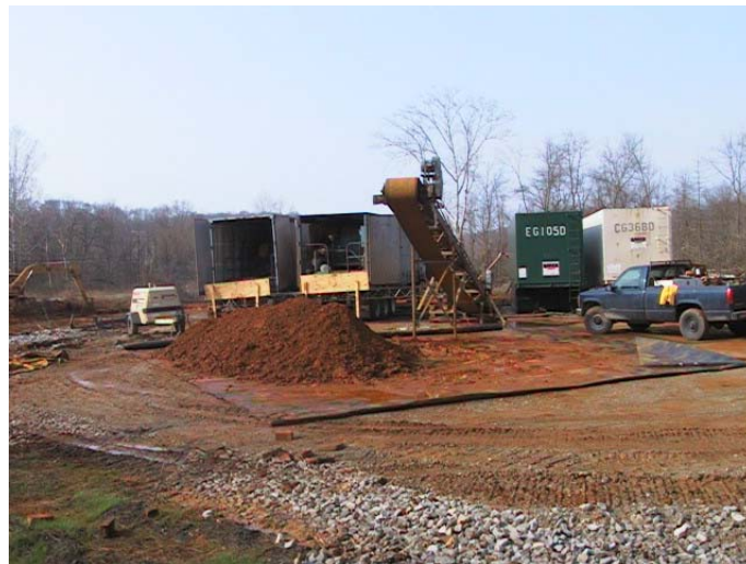
Figure 6. The two sludge storage tanks (right), two frame filter presses (left), conveyor, and product.
